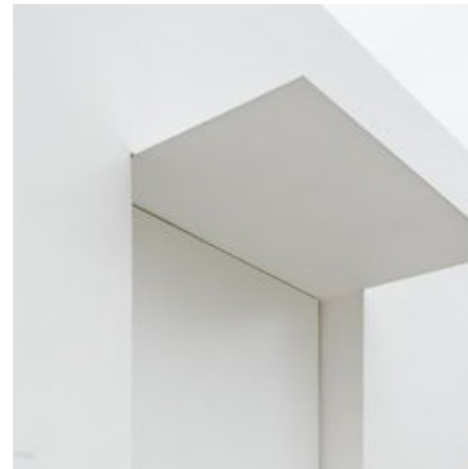
9. Pressed and powder-coated aluminium hoods over doorways and glazing provide adequate shading.
