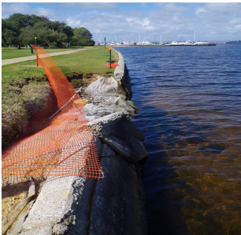
Figure 1 - Collapsed section of river wall (October 2016)
