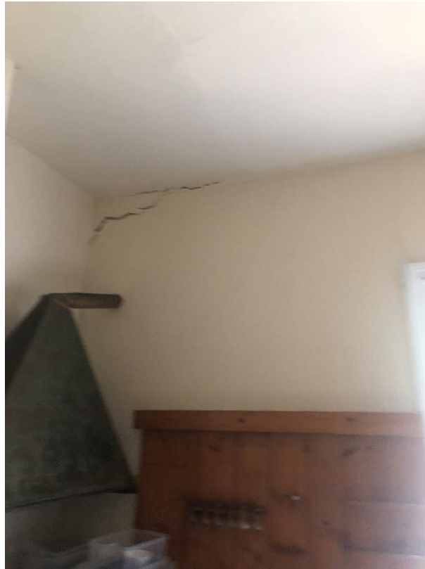
Photograph 7 – Cracked Plaster Wall-Kitchen
