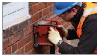
1. Rake out or cut slots into the horizontal mortar beds, a minimum of 500mm either side of the crack
