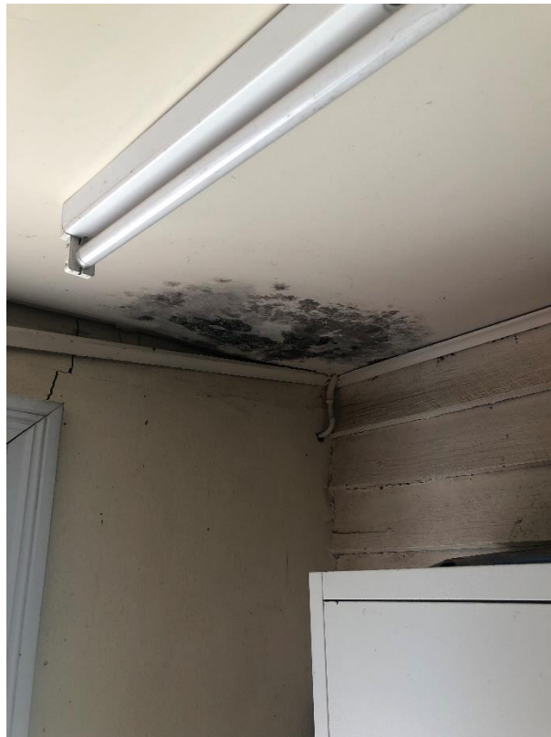
Photograph 8 – Water Damage to Ceiling
