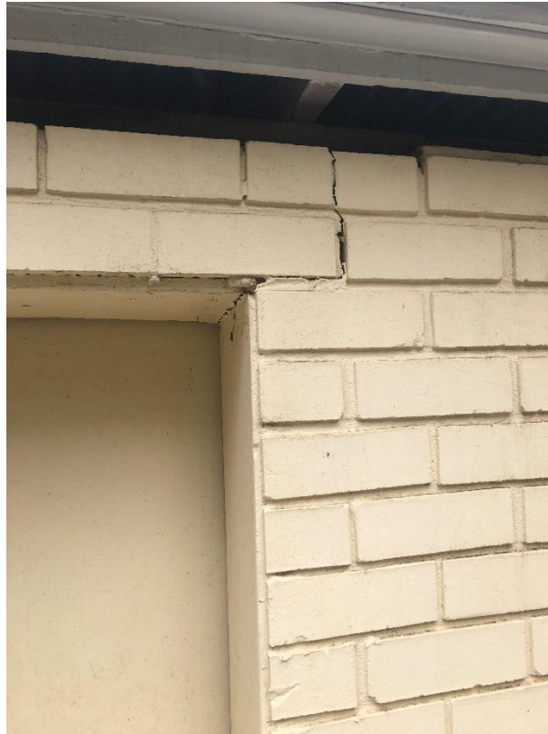
Photograph 3 – Masonry Wall-Cracking Above Door Opening
