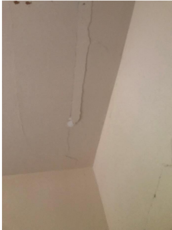
Photograph 9 – Cracked plaster Ceiling – Dining Room
