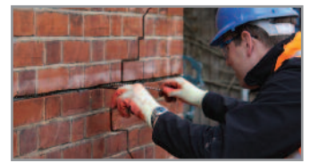
4. Using the HeliBar Insertion Tool, push one HeliBar into the grout to obtain good coverage
