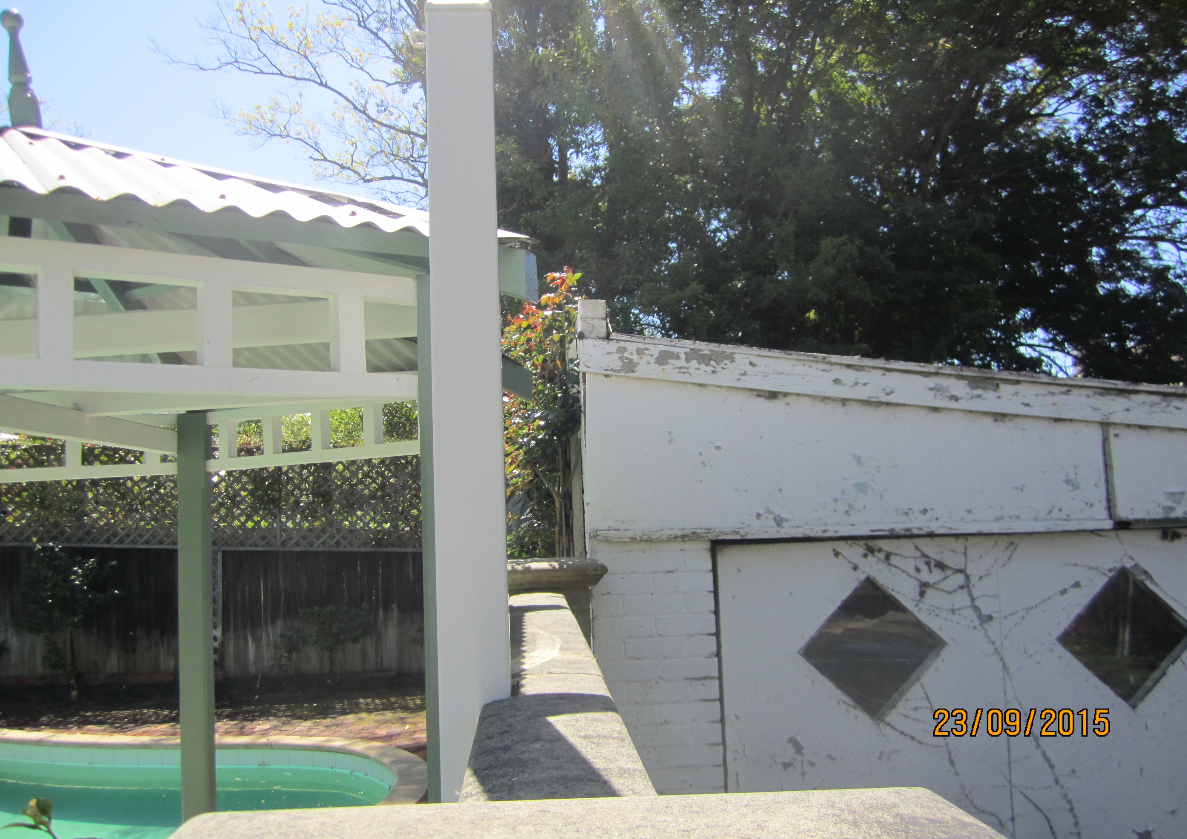
PD52.15 Attachment 6 - Photograph of existing garage parapet wall along the dividing boundary
