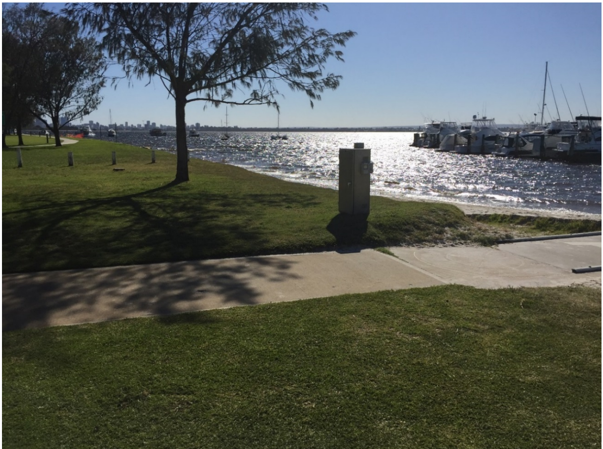
Services cabinet at northern entrance to the public access foreshore adjacent to the Club's lease premises
