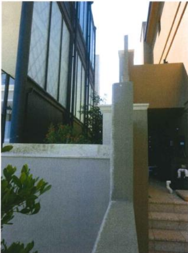
Photograph 4: Parapet wall created by the enclosure of pool equipment. The parapet is located below and behind the dividing fence between the subject site and No. 132 Victoria Avenue and is not visible from the adjoining property. Photograph also shows the extent of retaining on No. 132.
