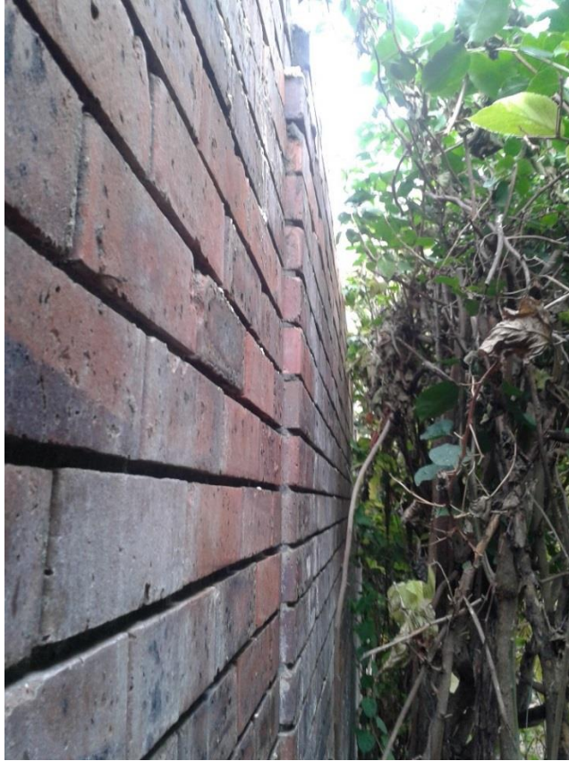
Neighbour (North) – Leaning Section of Side Fence
