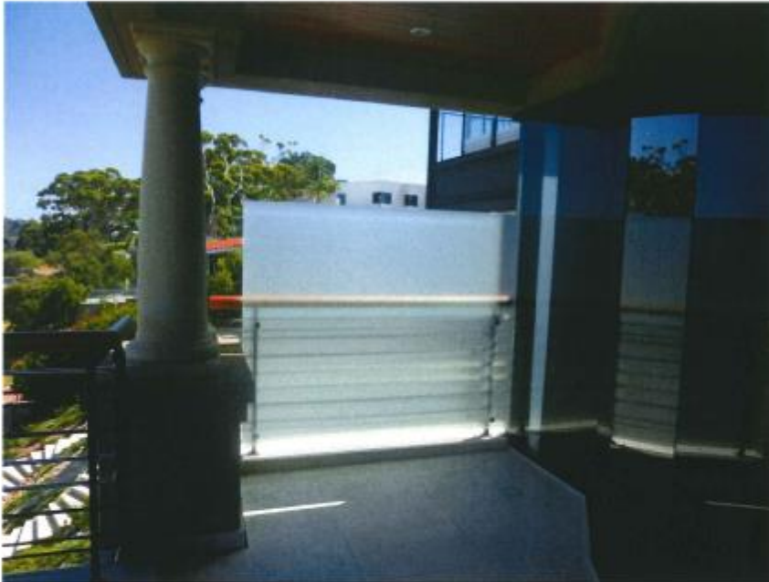
Photograph 7: All openings along the ground floor, where located more than 0.5m above NGL, are screened. This 1.65m high obscure screen is fitted to the ground floor balcony.
