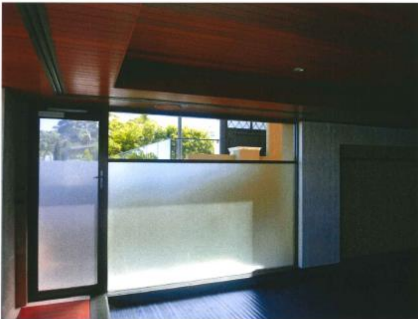
Photograph 5: The 'open' portion of wall has been fitted with a 1.65m high obscure screen to restrict any overlooking of the outdoor habitable space on adjoining No. 132 Victoria Avenue from the outdoor habitable space on the subject site.
