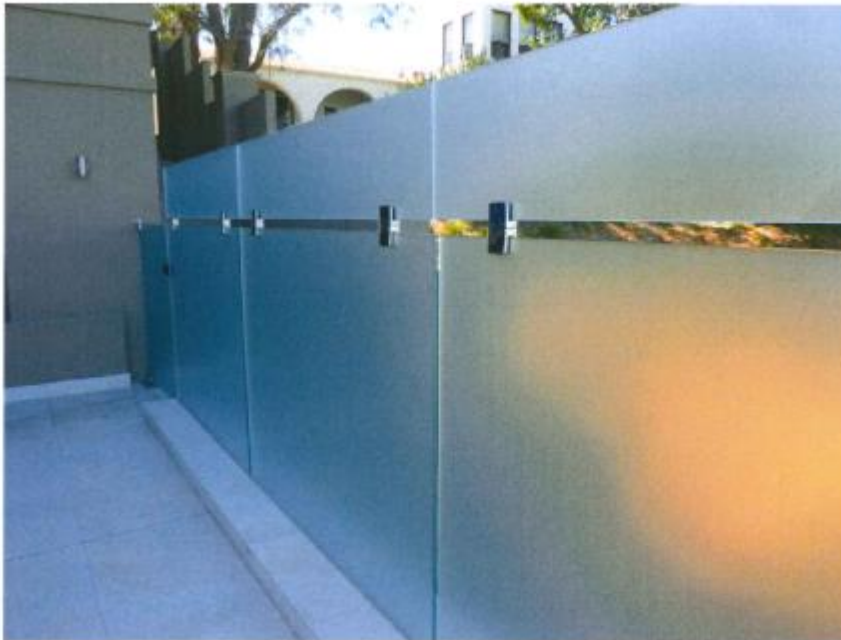
Photograph 3: 1.65m high obscure screen located along the southern boundary of the Uncovered Outdoor Living Area.
