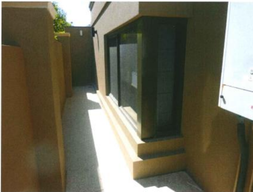
Photograph 6: A non-compliant portion of wall is partially located below NGL and is located behind and below the height of the dividing fence between the subject site and No. 132 Victoria Avenue.
