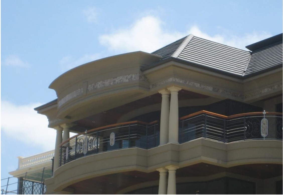
Site – Unauthorised Roof Extension over Upper-Rear Balcony
