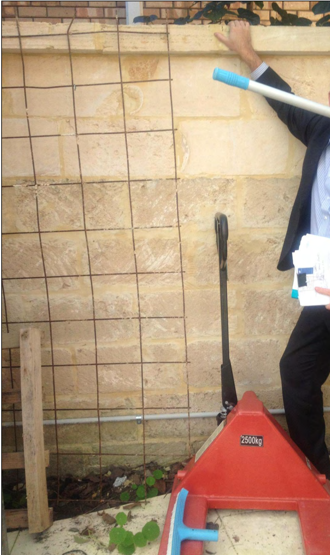
Over-Height Dividing Fence above Land Fill (North)
