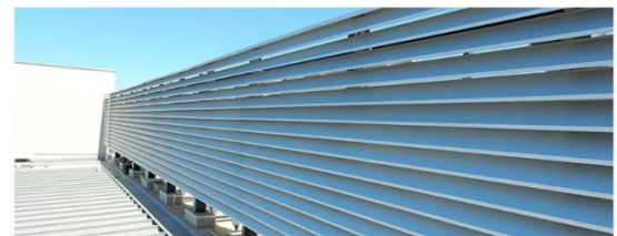
Typical Roof Mounted Condenser Screening
