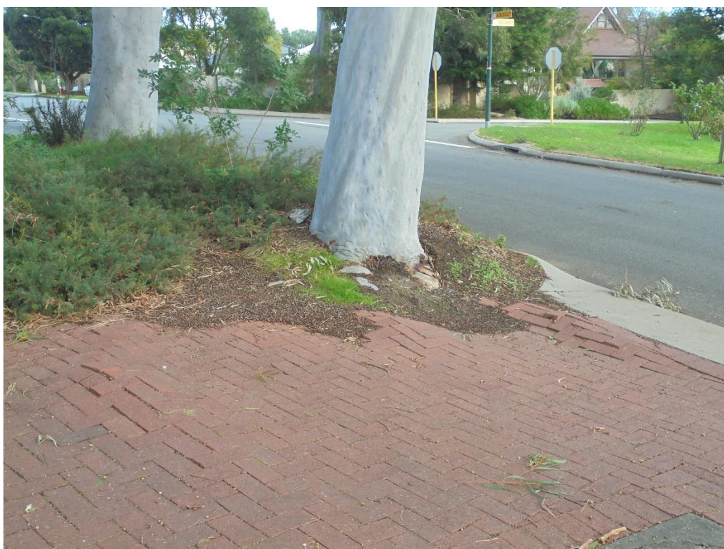
Figure 4 Displaying the base and lower trunk of Tree 2 viewed from the eastern side with lifting of adjacent paving evident.
