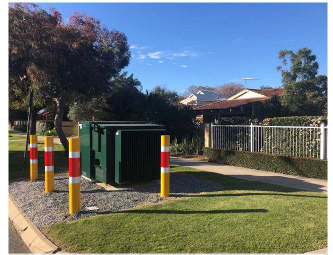
FIGURE 32 - EXISTING ELECTRICAL KIOSK
