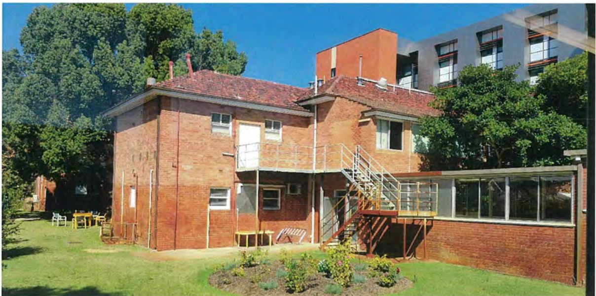
Old Building stock Circa 1940s – to be demolished near term Face brick
