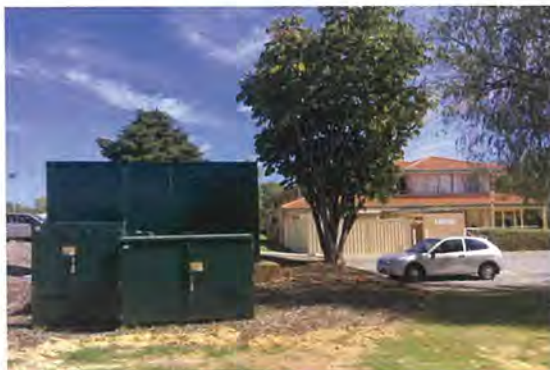
Transformer along William Road, to be screened with fencing.
