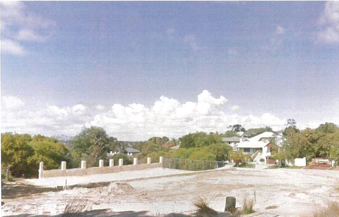
Figure 2 – Adjoining Strata Lots 1 & 2. Fill and retaining had been undertaken at subdivision stage.
