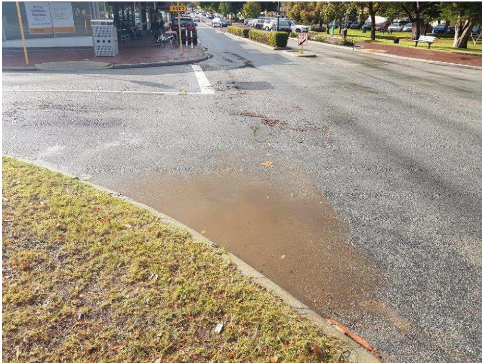
Figure 7 - Finding 4.5 – Drainage Deficiency
