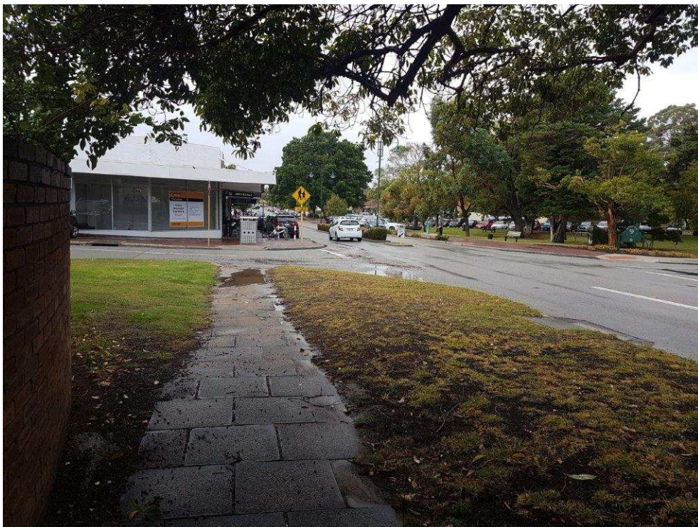
Figure 6 - Finding 4.4 – Footpath Condition
