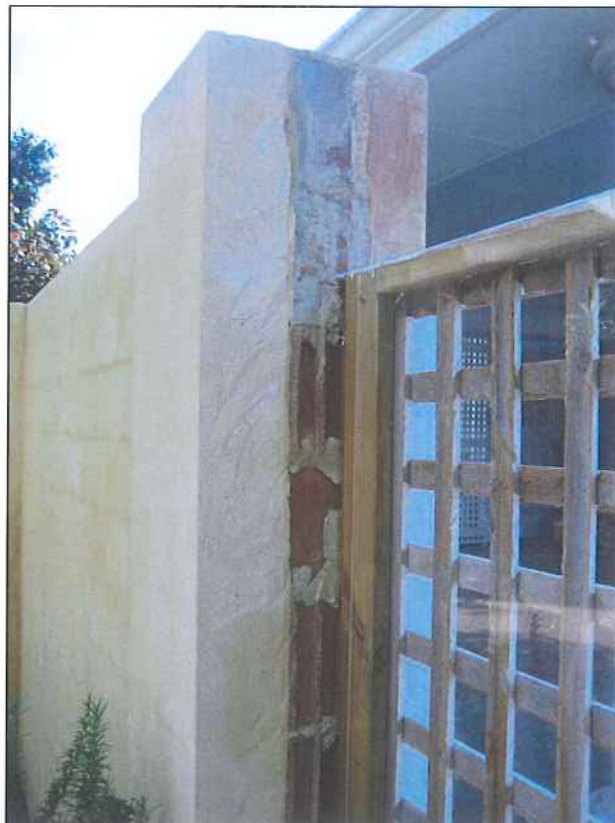
Unfinished Surface (bare maxi-bricks on the neighbour's side)
