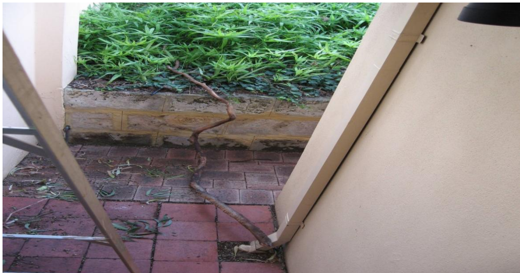
Figure 3 – Branch alleged to have caused the damage to the property (15 August 2011).
