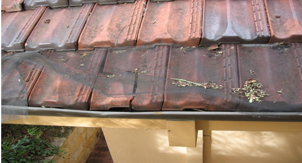
Figure 2 - Damage to tile, guttering and fascia board to property at 73 Melvista Avenue allegedly caused by falling branch from verge tree (15 August 2011).
