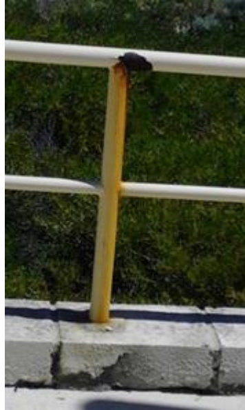
Figure1: Example of corrosion in existing handrail
